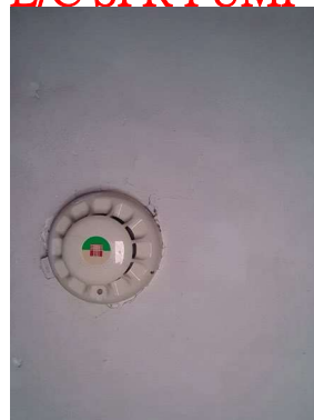
L/C SPR PUMP RM F5
