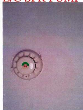
L/C SPR PUMP RM F5
